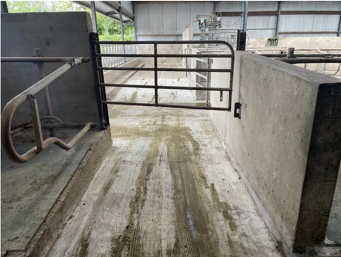
Fig 7. Raised gates requiring specific fabrication to facilitate scraper movement
