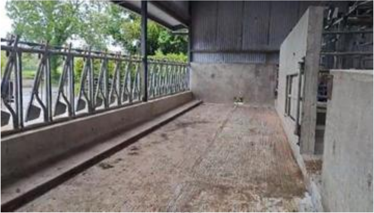
Fig 2. New passageway laid complete with step to guide scraper (near feed barrier)
