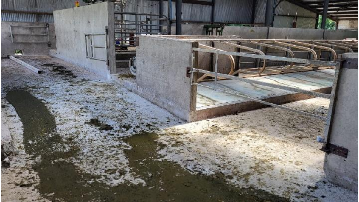
Fig 3. New passageway demonstrating the change in height and significant changes needed to accommodate the scraper.
