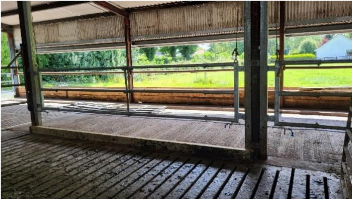
Fig 5. Passageway separated via installed barrier bolted to plates welded into place to reduce the size of the passageway.
