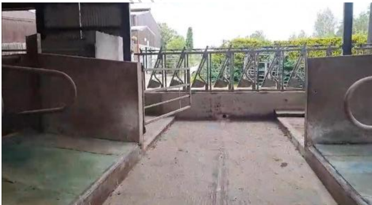
Fig 1. Existing passageway with steps to either side. These had to be removed and entirely new concrete passageways laid
